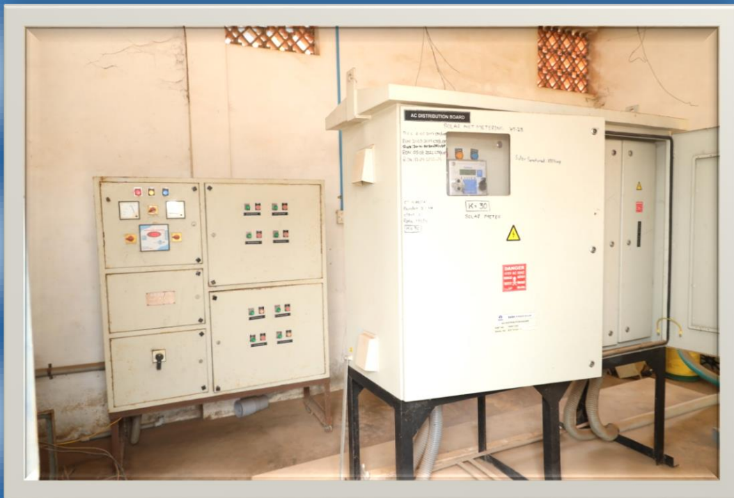
POWER CONTROL ROOM
